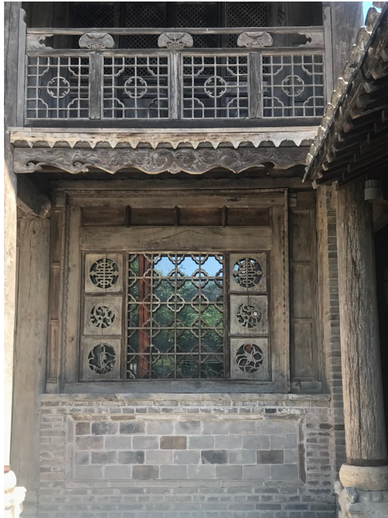
Figure 2.5: A distressed building using old wood and stone in Wuzhen. Photo by author.
